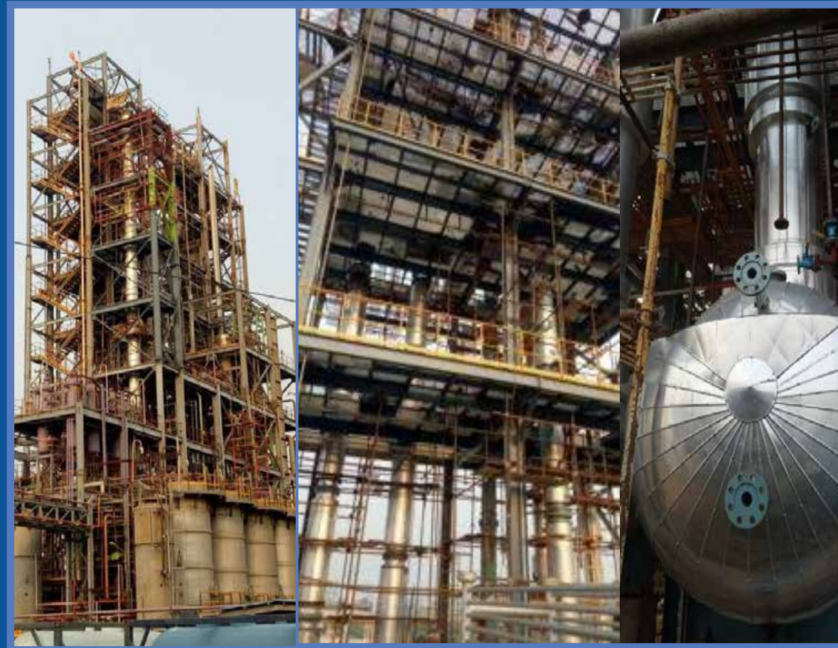
GFL , Dahej 10 Column Solvent Distillation Plant
