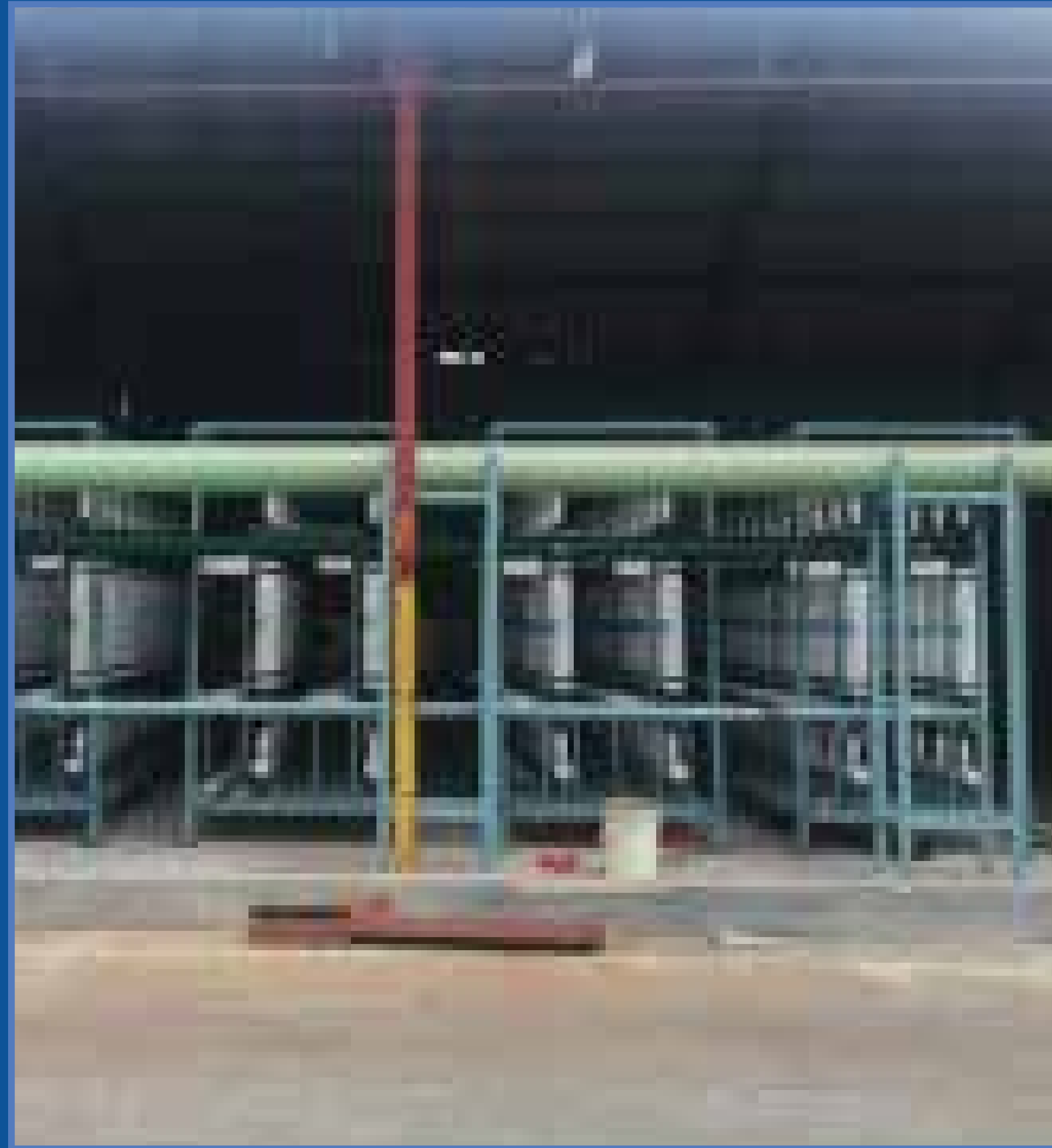
Recron Sdn. Bhd. Malaysia 5 MLD Ultrafiltration Water Treatment Plant
