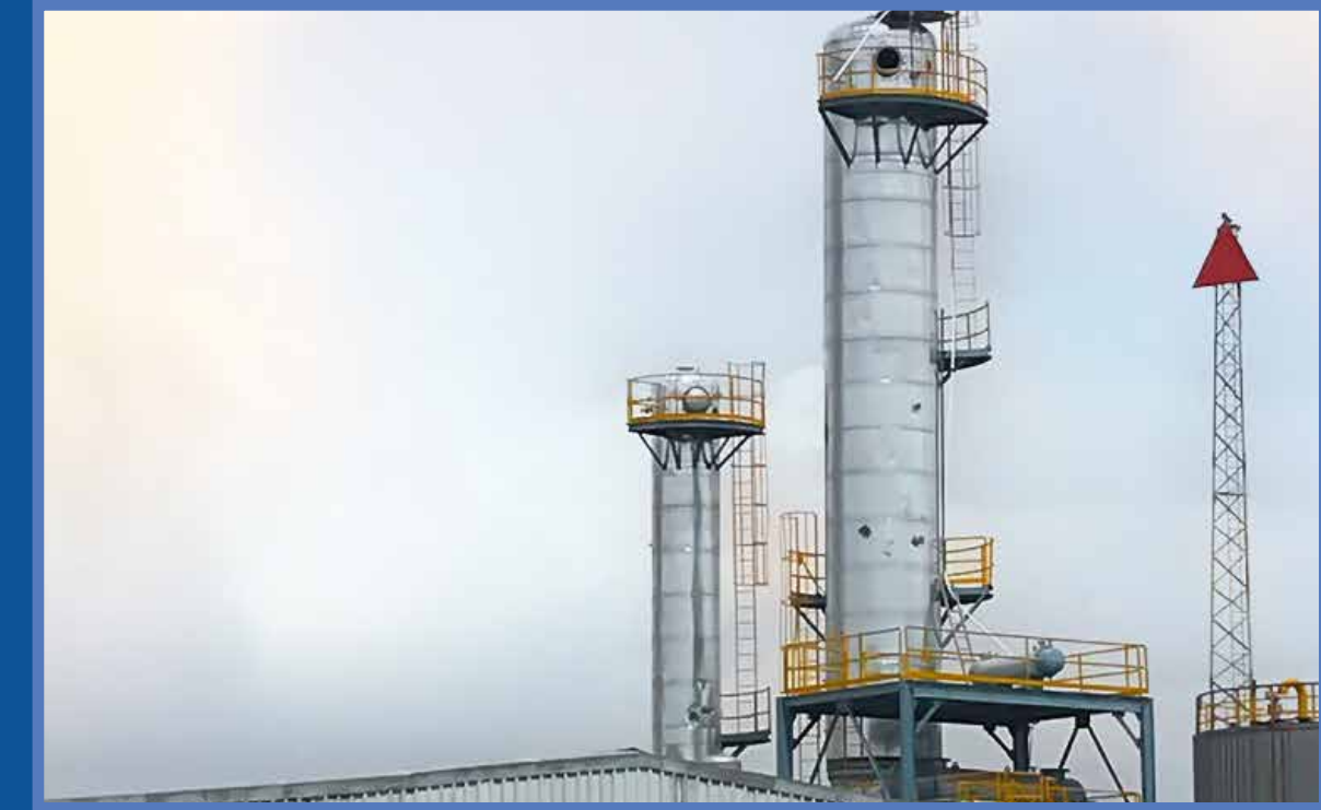
Taco Chemical , Turkey 100 TPD Ethyl Acetate Plant
