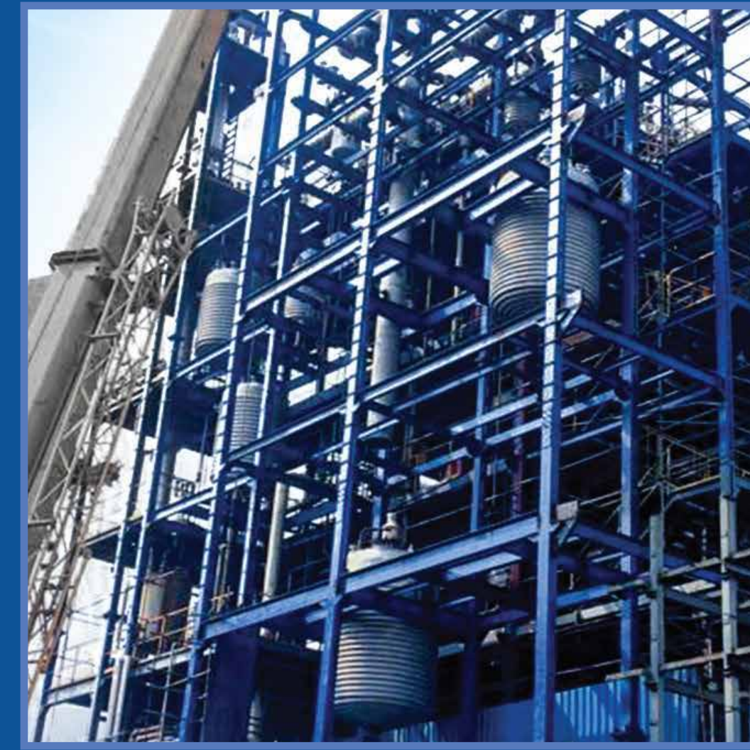
Laxmi Organic Industries (Reactor)
