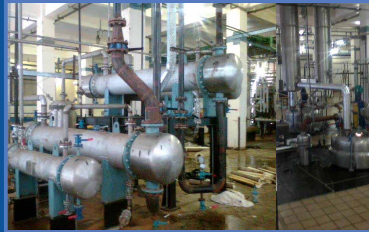
Rallis , Dahej 2 Stage Distillation Turnkey Plant
