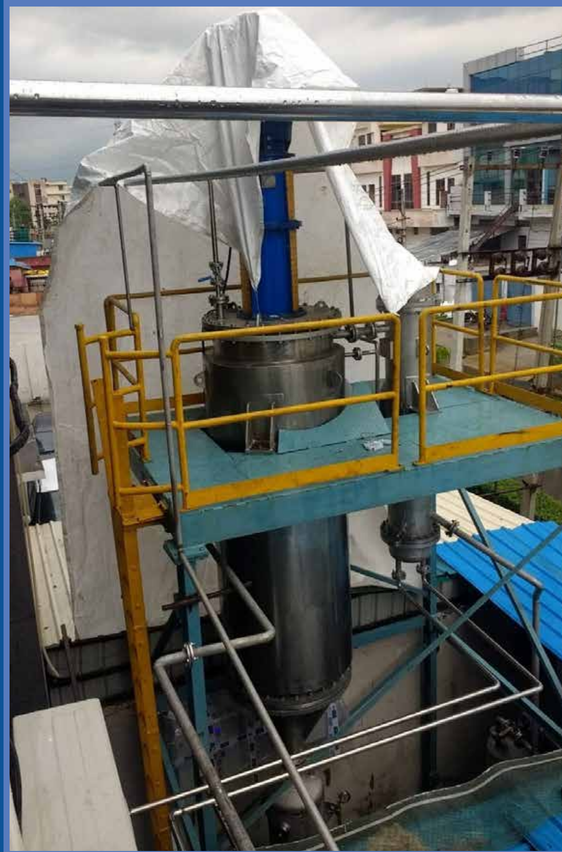
Jivo Wellness ATFD Plant
