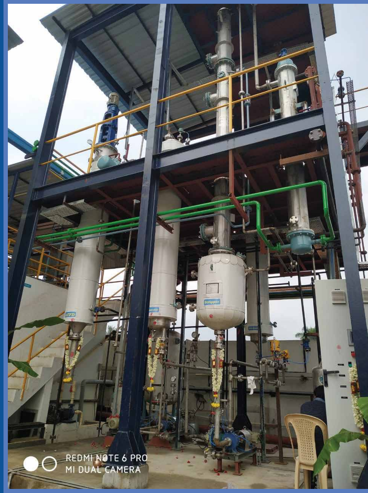
Hikal Limited Zero Liquid discharge System
